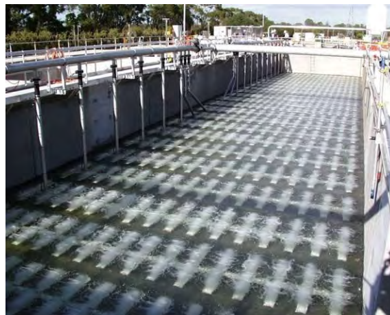
Oxley Creek bioreactor aeration system
