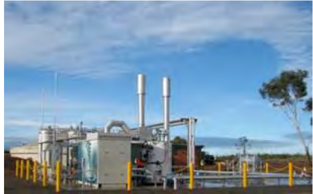
Biogas co-generation plant
